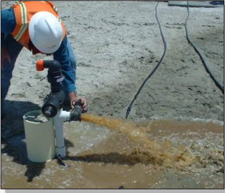
Opening flush manifold on Ram HWD system in Eastern California
